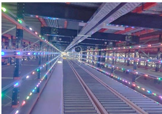
Fig.1. Warehouse using Pick-to-Light and Put-to-Light systems [4].
